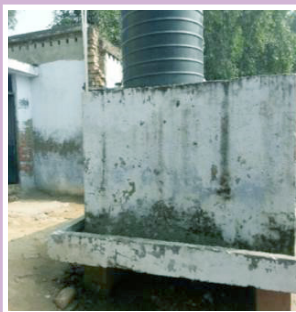
Sample Toilet (before intervention)
